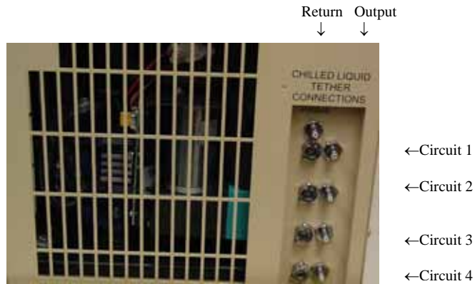
Figure 3 (Four person Chiller)
